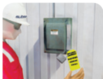
Lock out tag out system
